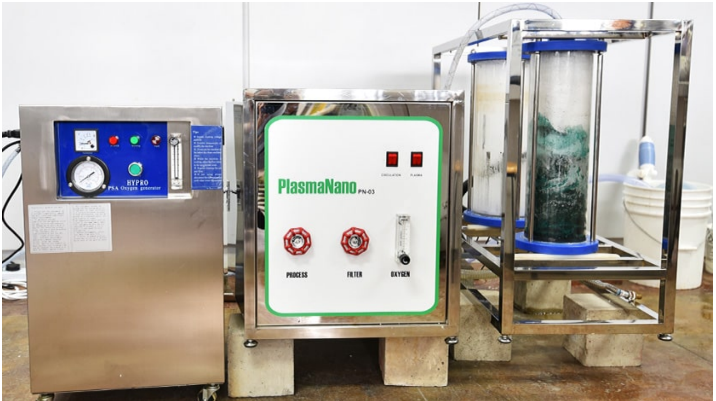
Samwoh’s wastewater treatment plant (Photo credit: Samwoh)
